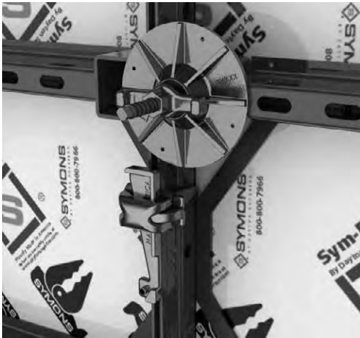
Clamp Adjacent to Tie Box
