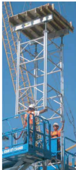
HV Support System Legs
