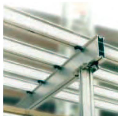
9. Position R12 x 100 and fix with a clamp at each intersection with a primary beam. Structure is now ready for fixing of plywood.
