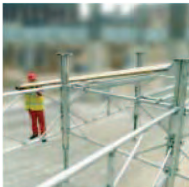
7. Place intermediate transoms and scaffold boards in position for fixing of alu beams.
